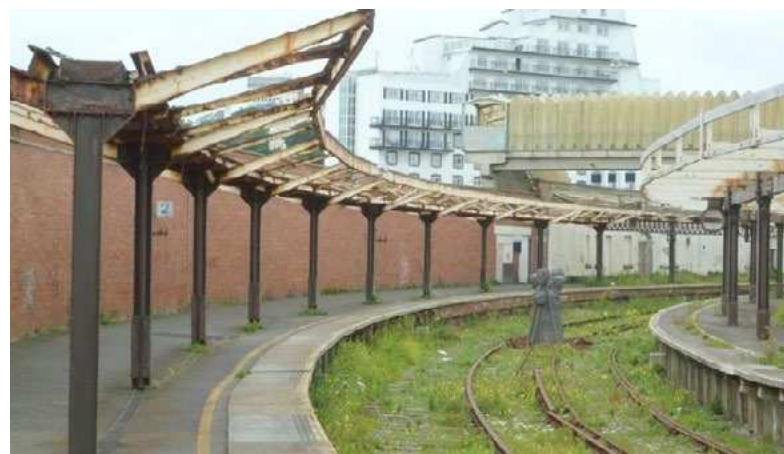
Fig 6.7.2 The dilapidated Harbour Station
