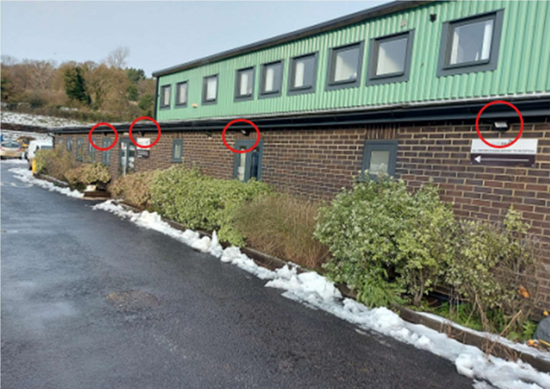
Image 5: Southern elevation – low level lights
