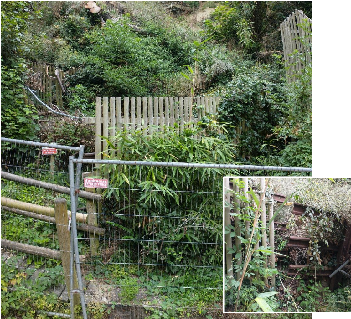
Photo 5. UC column fence with attached timber cladding moved due to slop. Small window shows sheared UC column pillar frame
