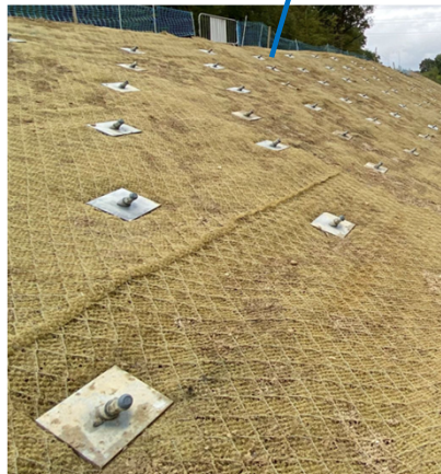
Soil nailing with steel mesh and erosion control blanket (Image taken from a Tony Gee project)
