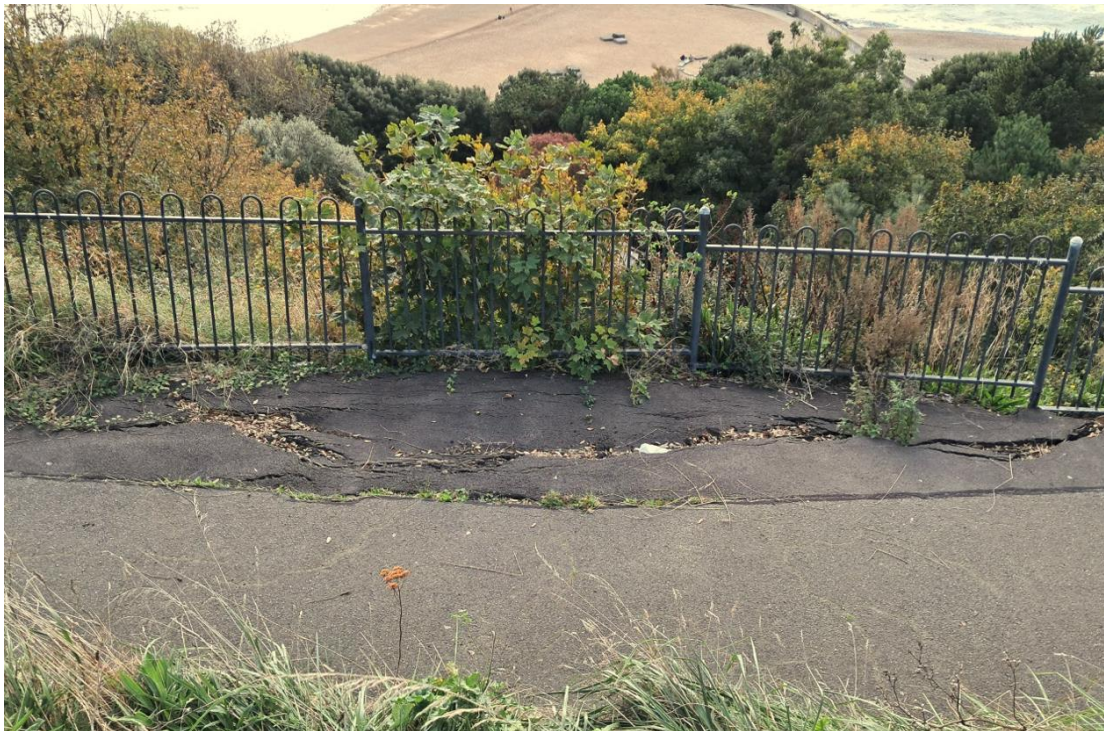
Photo 2. New cracks at the crest of the cliff shortly before the landslide. The pavement was repaired when the cracks first appeared (photo taken during our site visit)
