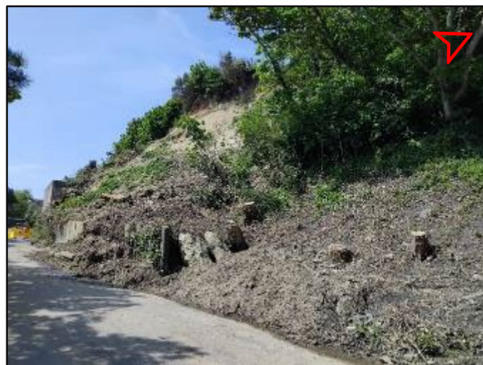
Photo 7 - Image showing the landslide / slip at the eastern extent of the Road of Remembrance.
