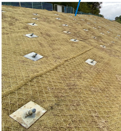
Soil nailing with steel mesh & erosion control blanket (Image taken from a Tony Gee project)
