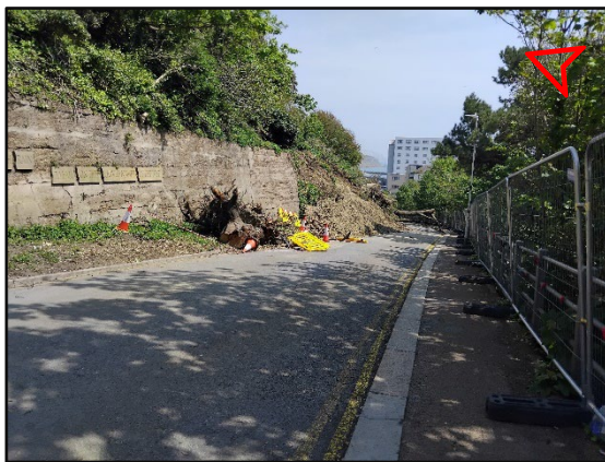
Photo 8 - Image showing the inclined retaining wall structure and western extent of the landslide / slip along the Road of Remembrance.
