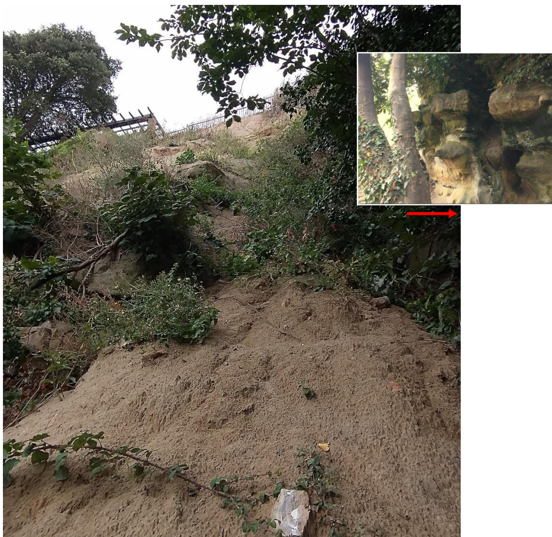
Photo 4. Slipped sandy material, with chert cobble and sandstone bands above. The window shows exposed sandstone blocks at the east (right) of this zone
