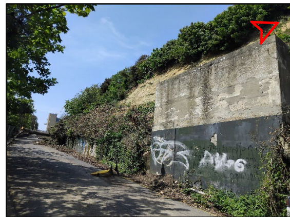
Photo 9 - Image of the landslide / slip above a small retaining feature / structure on the northern side of the Road of Remembrance and disused unknown structure.
