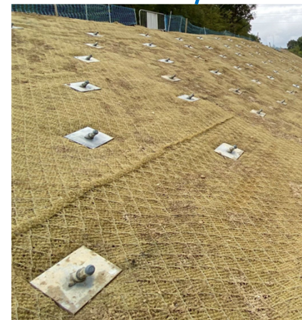
Soil nailing with steel mesh and erosion control blanket (Image taken from a Tony Gee project)
