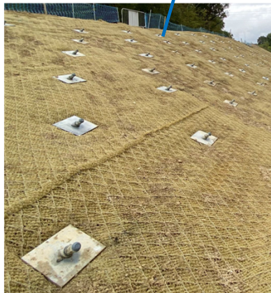
Soil nailing with steel mesh and erosion control blanket (Image taken from a Tony Gee project)
