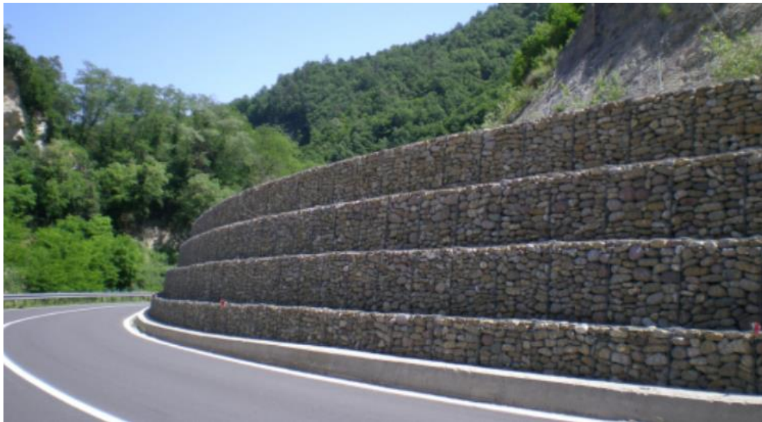
Photo 7. Gabion wall in front of a cliff (image taken from Maccaferri's website)
