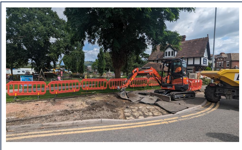
Here we are breaking out redundant footways by Radnor Park roundabout, these will be replaced with new materials.
