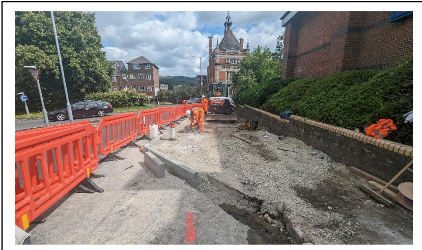
There is now one lane of traffic along Shellons Street, here you can see where we are in the process of widening the footpath for a safer pedestrian crossing.
