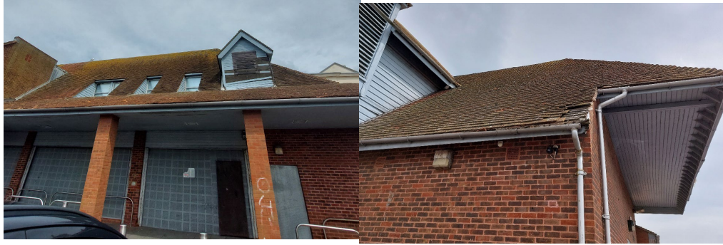
Image 03 – Example of damaged weatherboard and missing roof tiles.
